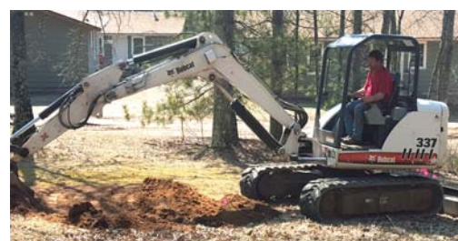
Soil testing begins on the site of The Bethel Family and Adult Retreat Center.
